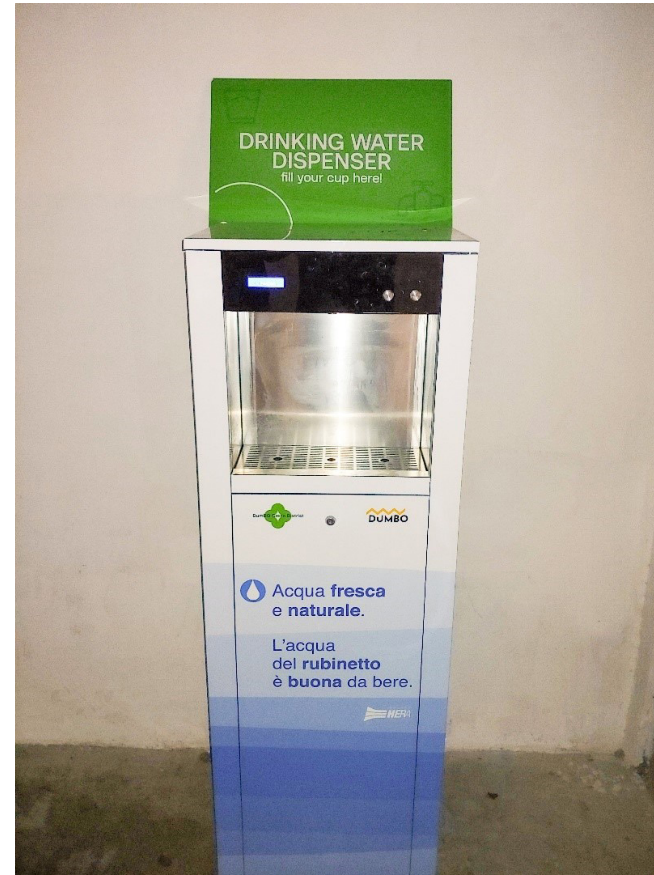
Photo 3. Micro-filtered drinking water tation installed inside one of DumBO's halls
